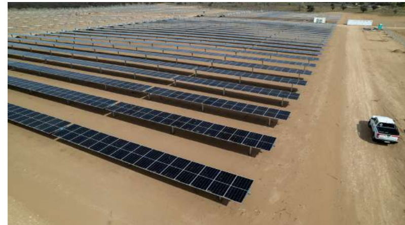
Photovoltaic Solar Power Plant in Victoria (7.2 Mw)
