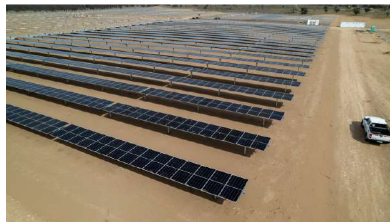
Photovoltaic Solar Power Plant in Victoria (7.2 Mw)
